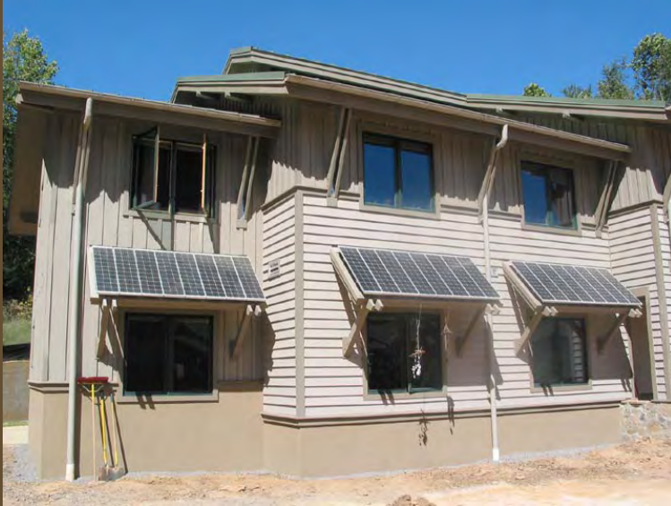
Solar PV panels on window overhangs
