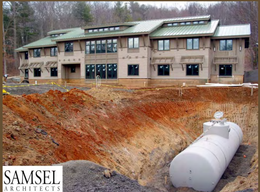
10,000gal rain water cistern
