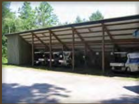
Golf Carts at Charging Station
