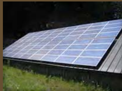
PV Panels on Charging Station
