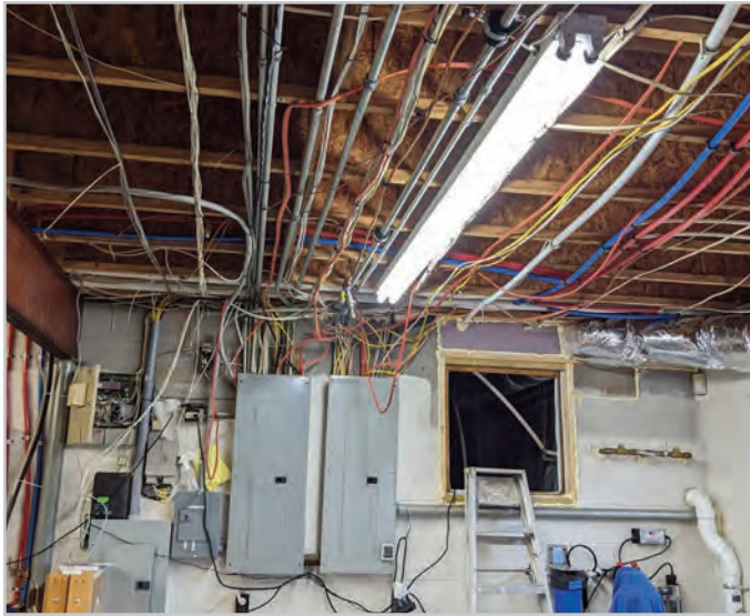
Disconnected cable wires can become a parallel neural pathway, causing high magnetic fields.
