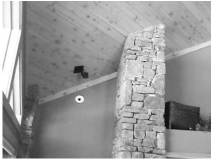
While under depressurization, cold air is pulled through holes in the envelope.
