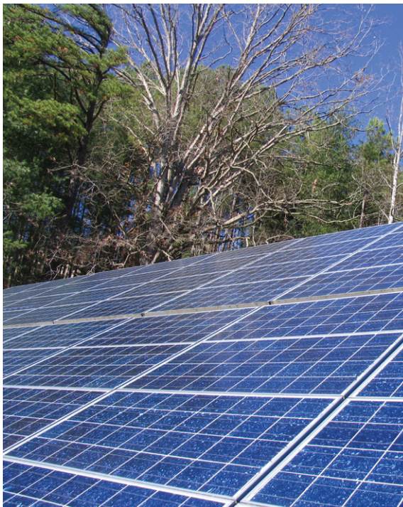
Solar electric panels mounted on a rooftop (photo by Rebecca Bowe).
