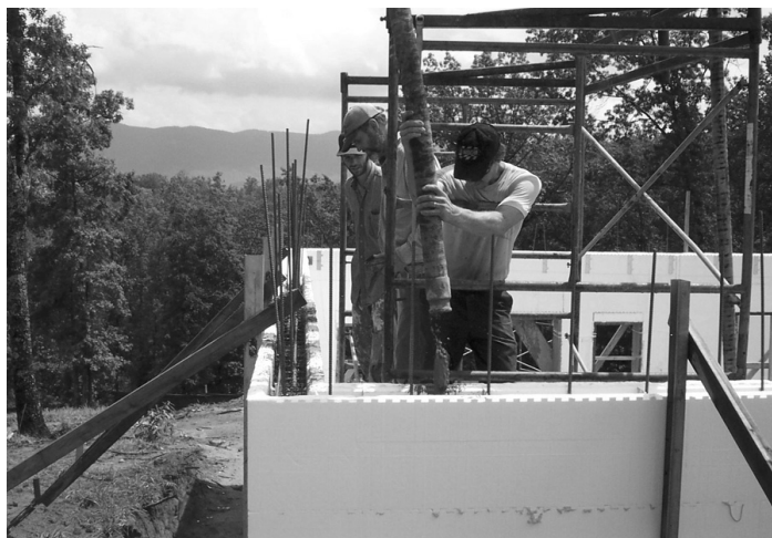
This ICF wall shows reinforcing steel inside before the concrete pour (photo by Marcus Renner).
