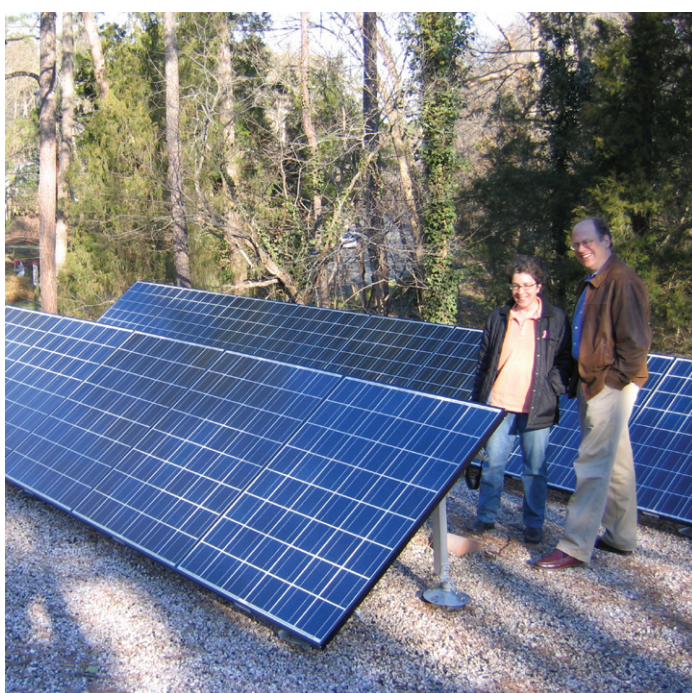
Residential 2.7 kW grid-tied PV system located in Durham. This project is part of the North Carolina Green Power Program, designed and installed by Sundance Power Systems in 2005 (photo by Dave Hollister).
