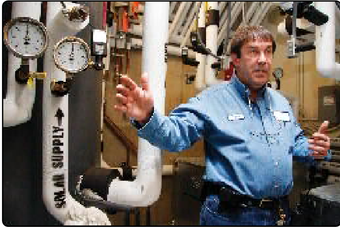
Tony Kapustka, HVAC mechanic at UNCA, says the building's solar and geothermal heating-and-cooling system is really quite simple.
