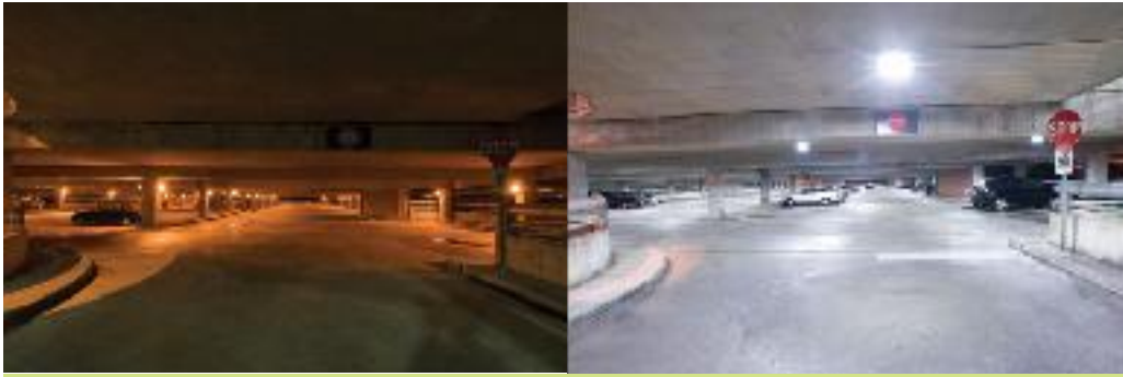
Before and after: At N.C. State University, the parking deck was lit by the dingy orange glow of high-pressure sodium fixtures (left); the new LEDs brighten the space and save 27 percent in energy costs.
