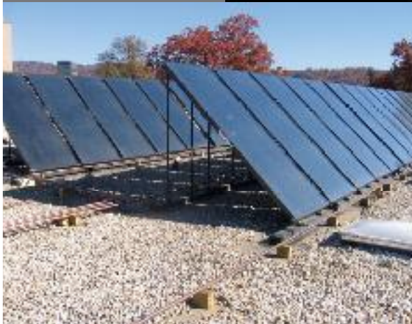
Solar thermal pool heating at YWCA in Asheville
