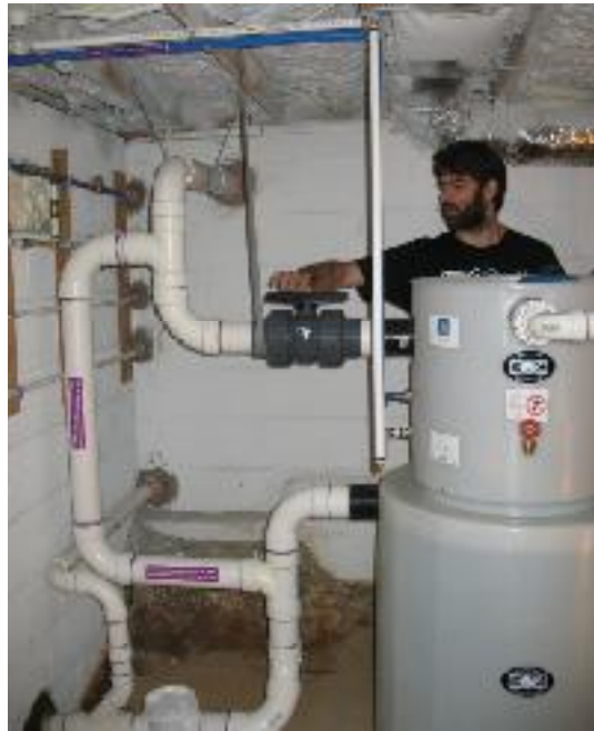
Get it approved: In North Carolina, all graywater systems must be approved by code officials prior to installation per job site. photo courtesy of A2Z Plumbing
