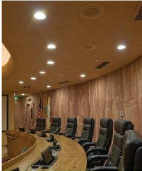
Lighting matters: At Indian Wells Town Hall, the conversion to Cree LR6 LED lights reduced electricity consumption by 80 percent. photos courtesy of Essential Systems Engineering
