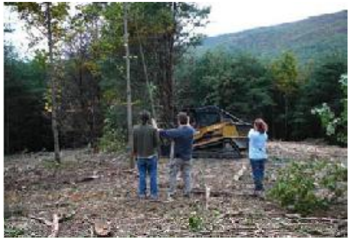
Half-way there: Sharapan and Haagensen look on as the site is cleared. Material is in "rough" phase.
