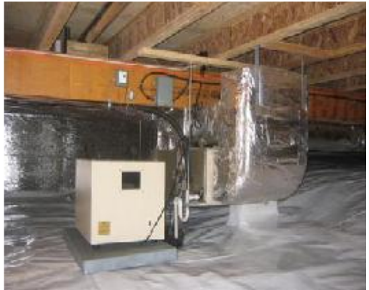
A clean start: Sealed crawlspaces are one effective method for getting HVAC equipment into the conditioned space.
