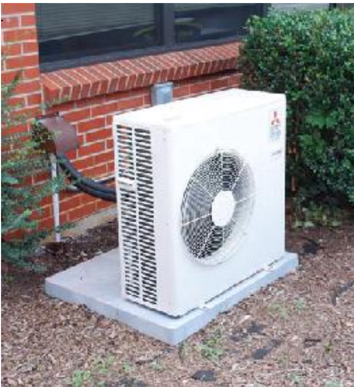
A better heat pump: Hot Springs Elementary replaced a failing central boiler system with classroom heat pumps, providing numerous performance benefits and energy savings.
