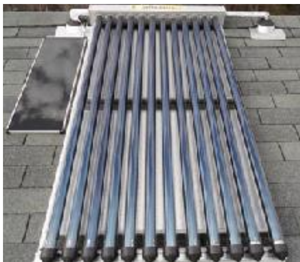
Solar thermal systems: This one, with evacuated tubes, can provide 75 percent of a family's hot water needs.
