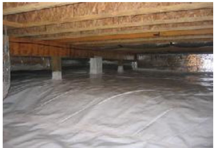
Sealed is better: Closed crawlspaces are a great moisture-control strategy and can reduce energy consumption.
