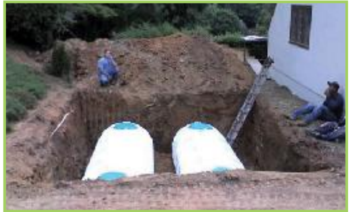
Size: 3,400-gallon below-ground system Use of water: Irrigation, especially grape vines Where: Nery residence in Beaverdam, Asheville, N.C. System installed by: A2Z Plumbing photo by Miranda Efird, A2Z Plumbing
