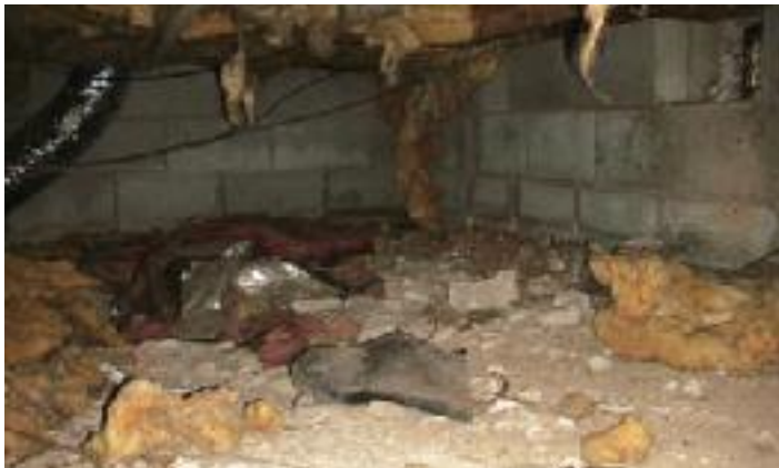
Problems galore: Vented crawlspaces can lead to mold and moisture problems.
