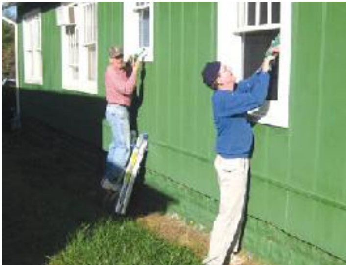
Good works: These volunteers are sealing the windows to prevent drafts and save energy PHOTOS COURTESY OF AMERICORPS RECOVERY PROJECT ENERGIZE
