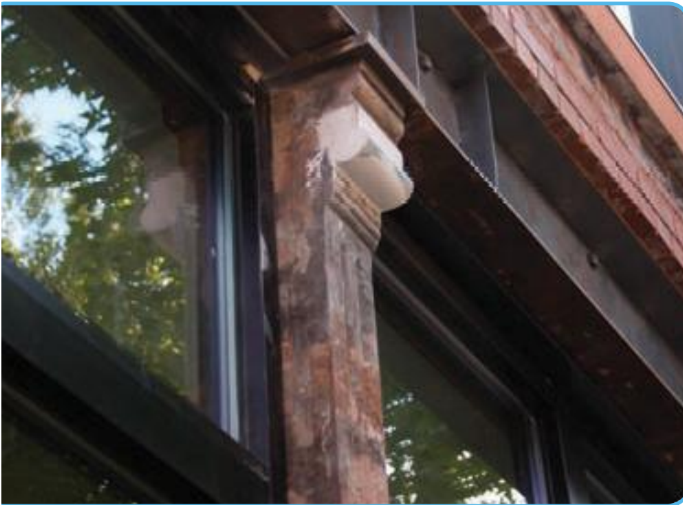
Uncovered: During the demolition stage, contractors discovered cast-iron support columns, embellished with floral designs. Such features hint at the building's early days at the turn of the 20th century.
