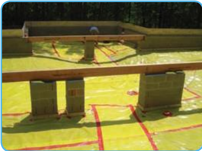
Details: Every step matters, from well-sealed crawlspaces to keeping the building site organized. photos by Jim and Kris Forward
