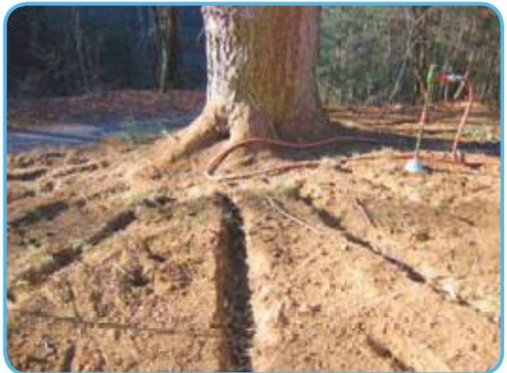
Tree saver: Radial trenching uses a compressed air gun to create a path for increasing aeration to a root zone.
