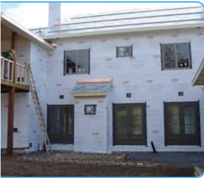
Wrapped up: Careful application of the housewrap helps ensure a tight home that will last for years.
