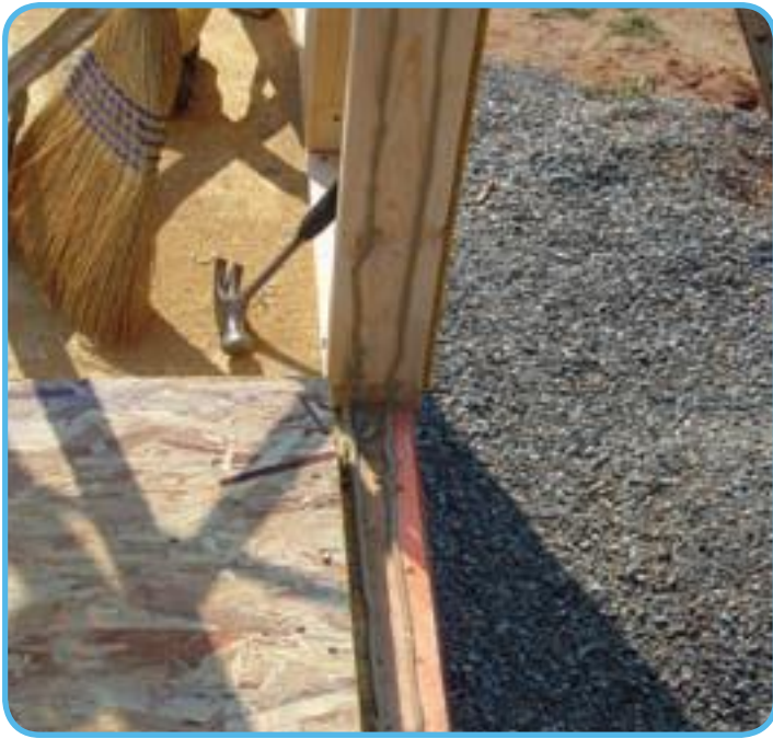
Good barriers: Gluing exterior walls can make the difference in creating a good air barrier.
