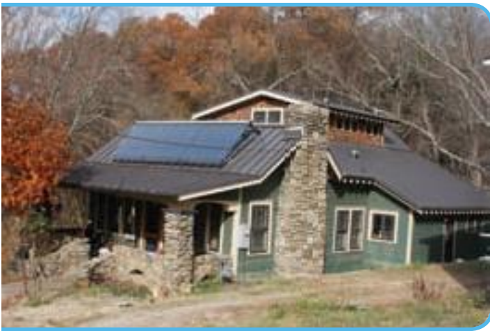
Gaining control: Water heated in an evacuated tube system on the roof provides radiant in-floor heat organized in four zones in the house, as Blake Esselstyn explains. Natural gas provides backup on cloudy days. Solar collectors, a second-floor addition, and original rock work are visible at this updated 1920s cottage.
