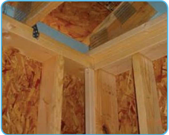
Details: Two-stud corners, raised-heel trusses and proper blocking are important construction details of ENERGY STAR home.
