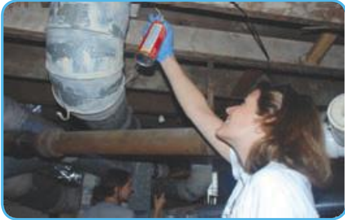
Energy saver: An AmeriCorps Member uses a can of spray foam to air seal large holes under the floor to save energy and improve comfort during "Project Energize."
