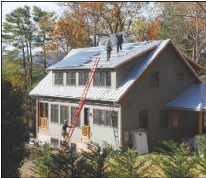
Score one for sustainability: Workers install PV panels that will help make the home net zero.
