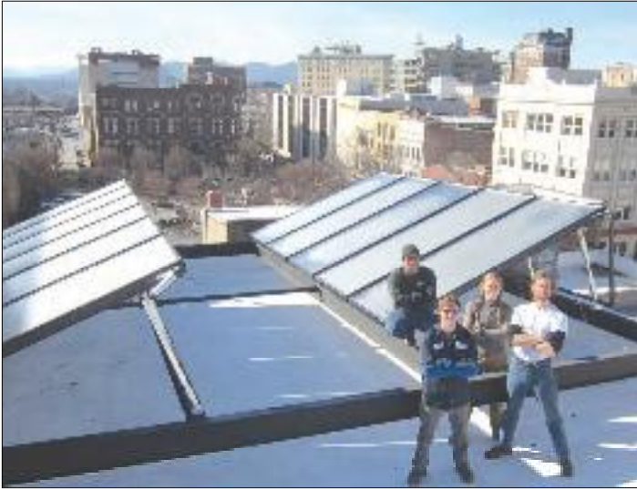
Sun team: Sundance Solar Systems helped the French Broad Chocolate Lounge and Posana Cafe get greener with these solar panels. PHOTO COURTESY OF SUNDANCE SOLAR
