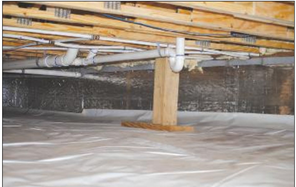
The good and the ugly: In the top photo, moisture has compromised the walls and subfloor. An improved crawlspace (lower photo) features a covered subfloor, insulation and other features.
