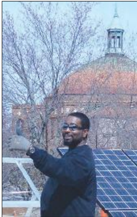
Thumbs up: Asheville's first community solar project resides on the roof of the First Congregational United Church of Christ.
