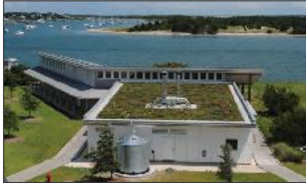
Hurricane-ready: The green roof on the Ocean Conservation Center at Duke University's Marine Laboratory in Beaufort, N.C., survived a direct hit from Hurricane Irene. PHOTO COURTESY OF DUKE UNIVERSITY
