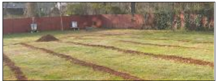
Figure 4: Piping laid out like a “vertical Slinky” is placed in trenches for this geothermal loopfield.
