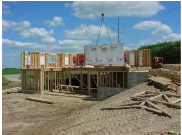
Pieces of the puzzle: Panelized homes are built quickly, which reduces on-site waste, protects materials from the elements and cuts labor costs.
