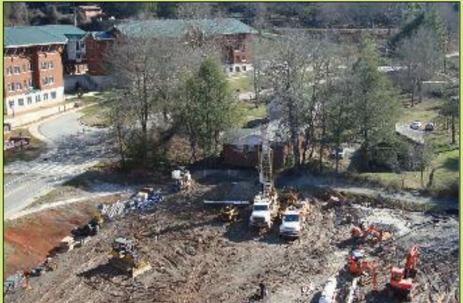
Earth warmed: While Warren Wilson College has earned national recognition for its green initiatives, other regional institutions have set to work too, such as this geothermal-well system under way at Western Carolina University.
