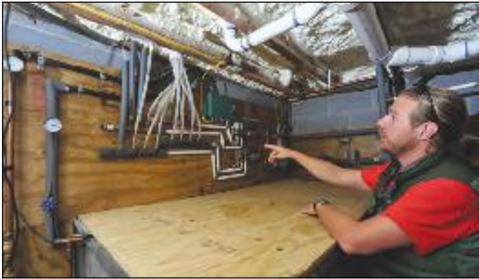
Systematic: A solar-thermal installation supplies the radiant-heat floor system, above, one of several features that help achieve net-zero energy use, says homeowner Ryan Lubbers.
