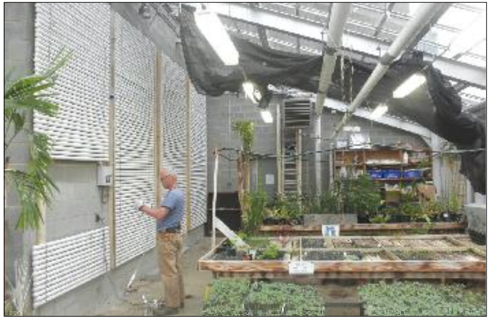
Hot and cold: Andy Reinhart installs PCM pipes at A-B Tech's Sycamore greenhouse. The thermal-mass system helps heat the greenhouse in winter and cool it in the summer.
