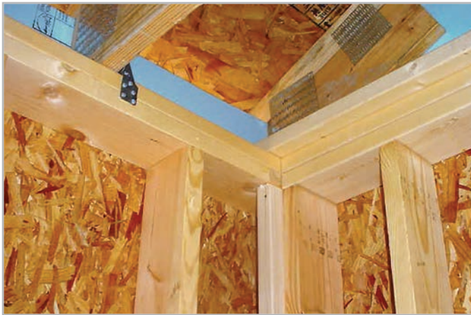
Advanced framing and blocking at Prospect Terrace, built by Mountain Housing Opportunities, the pilot project for NC Healthy Built Homes (now Green Built NC).
