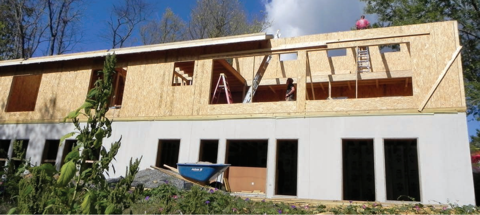
Structural insulated panels (SIPs) on a Superior Wall foundation for a passive solar home. VandeMusser Design photo
