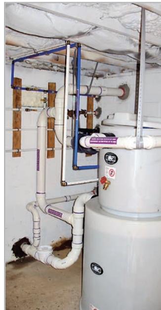
Greywater plumbing. Georg Eifird, A-2-Z Plumbing photo
