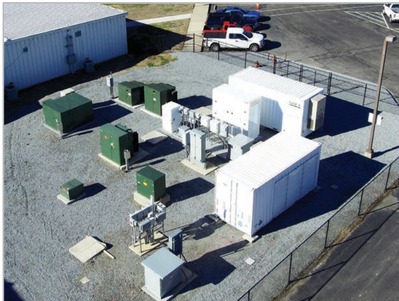
The Mount Holly Microgrid project located in Gaston County features a Saft 650kW lithium-ion battery and a 200kW Alevio lithium-ion battery. The battery storage system is integrated into a microgrid with more than 115kW of solar panels. In addition, residential energy storage systems from Tesla and Enphase are being tested and providing valuable insights into future benefits and operational realities of behind-the-meter energy storage. DUKE ENERGY PHOTO
