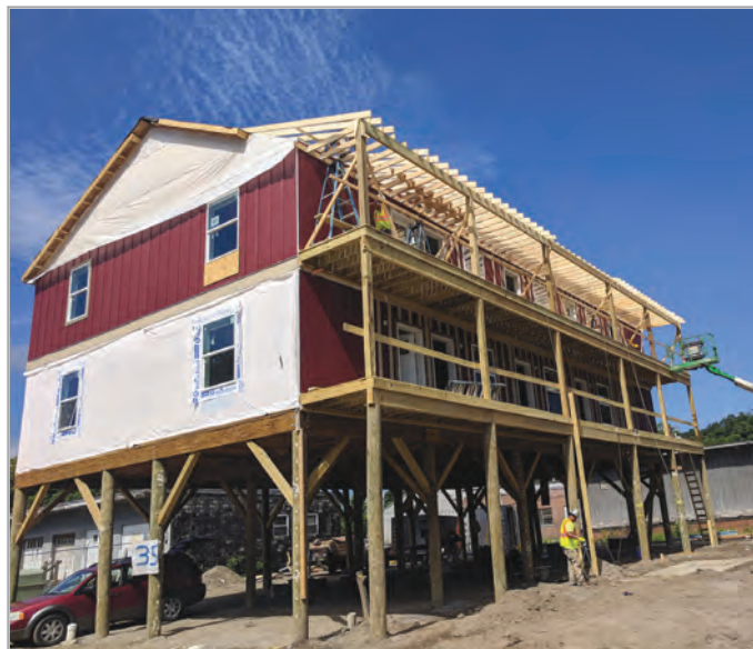
A 70-unit private-sector affordable housing development is now under construction in Asheville by Swannanoa Bend LLC. The City of Asheville is providing loan funds from its Housing Trust Fund, as well as a Land Use Incentive Grant. PHOTO COURTESY OF KIRK BOOTH
