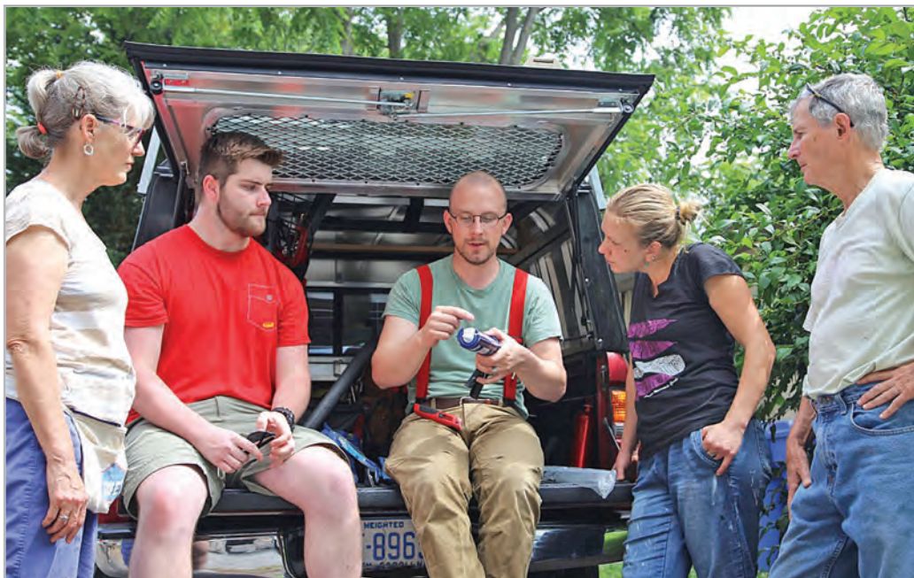
Above, Energy Upgrade Program Manager Jonathan Gach goes over tips for using a caulking gun with volunteers from Energy Savers Network during a workday at a local low-income home. At right, Gach installs weatherstripping on the front door of a local low-income home. DAYNA REGGERO PHOTOS
