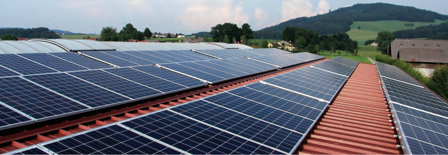
A raised-seam metal roof was determined to be the best solution for attaching solar panels and providing a clean platform for rainwater harvest.
