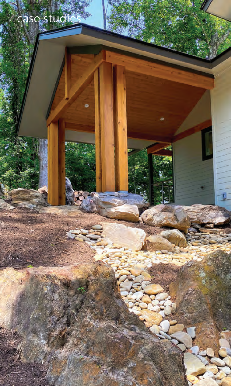
Six large cedar posts were mounted on top of two large boulders to carry the welcoming entry gable, creating the effect of the house coming right out of the rocks. RS MOTLEY CONSTRUCTION PHOTOS
