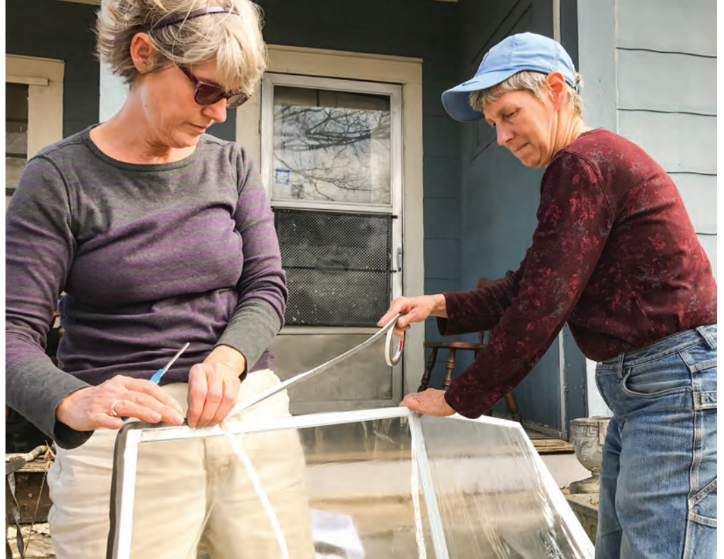
Energy Savers Network Co-Founder Alice Wyndham and Susan Presson work on building the first interior storm windows outside a client's house in 2017. BRAD ROUSE PHOTOS
