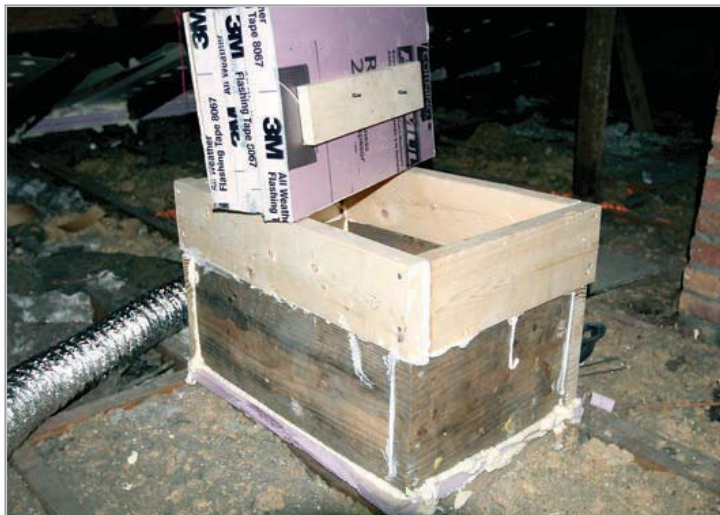
A well-insulated attic door and attic insulation can cut heating costs by half.
