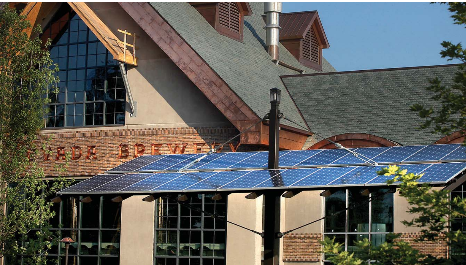
Solar panels at the Sierra Nevada Brewing Co. facility in Mills River.
