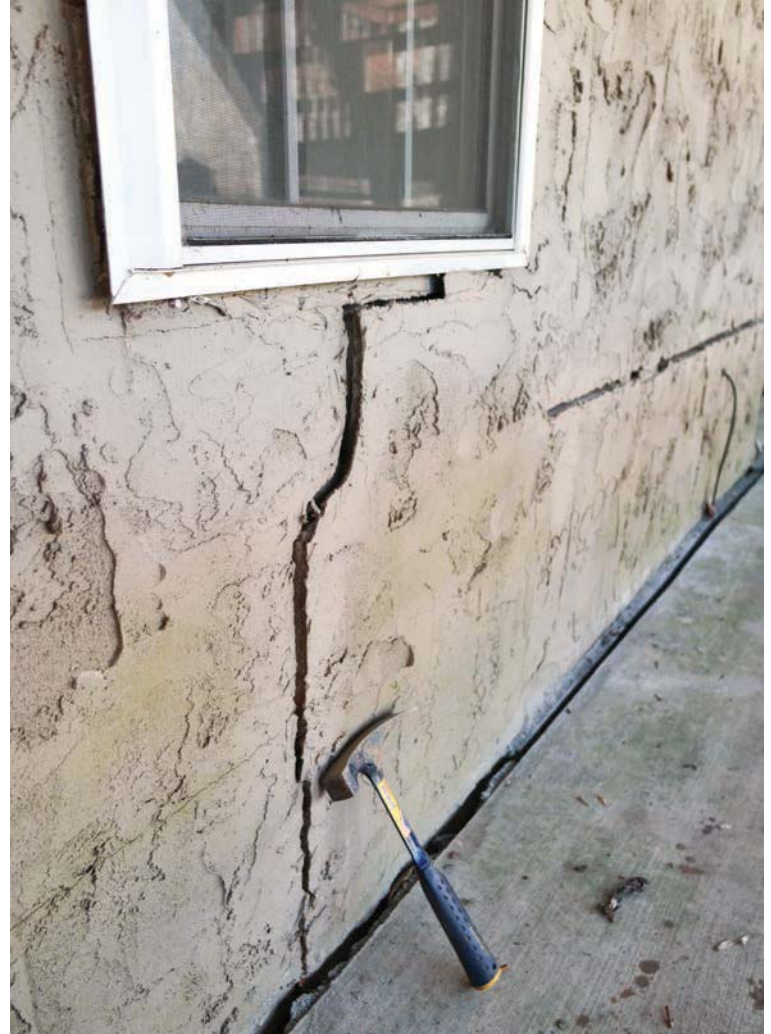
Cracks in the home foundation. Photo by Appalachian Landslide Consultants, PLLC
