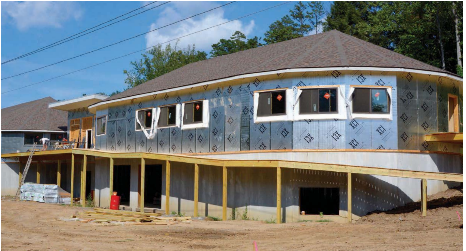
Located in the Riverside Business Park in Asheville, the future home of the French Broad River Academy is currently under construction. Utilizing renowned structural components and designs from Deltec Homes in Asheville, the school will not only have optimum functionality, it will also have the highest standard of green building materials for an eco-friendly and economical alternative to traditional building methods. Garret K. Woodward photos
