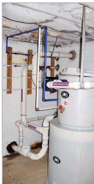
Greywater plumbing. Georg Efirid, A-2-Z Plumbing photo
