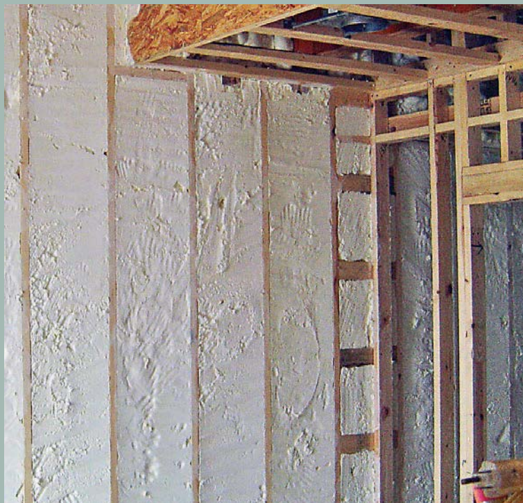
Ladder T wall's use scrap wood as a nailer for drywall and increase the amount of insulation at every interior-exterior wall intersection.
