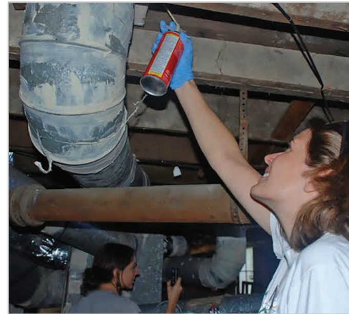
Sealing leaks around ductwork improves efficiency. Donated photo
